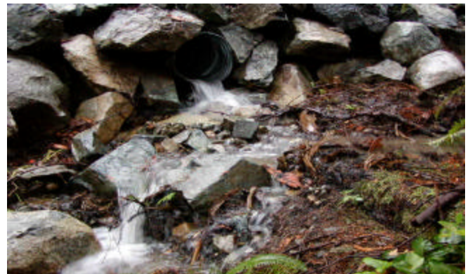
Culvert discharge 2 l/s with turbidity of 100 ntu. This represents 400 mg of sediment per second.
